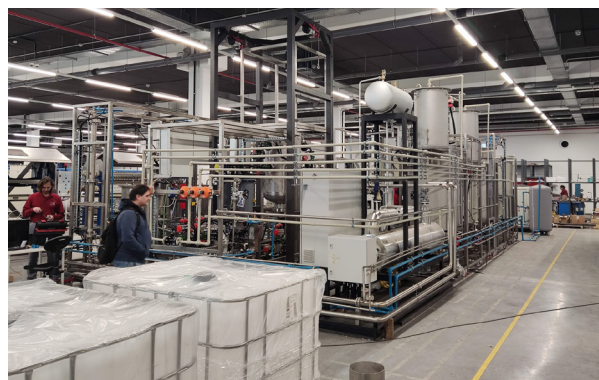
General view of the ICP pilot plant during its final assembly phase.
